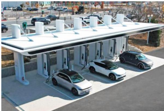
Hyundai EV charger installed at a public owned parking lot
